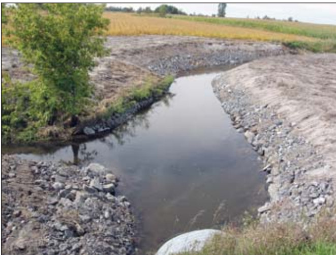
Photo 9: Protection upstream of the culvert Source: Mikael Guillou, MAPAQ
