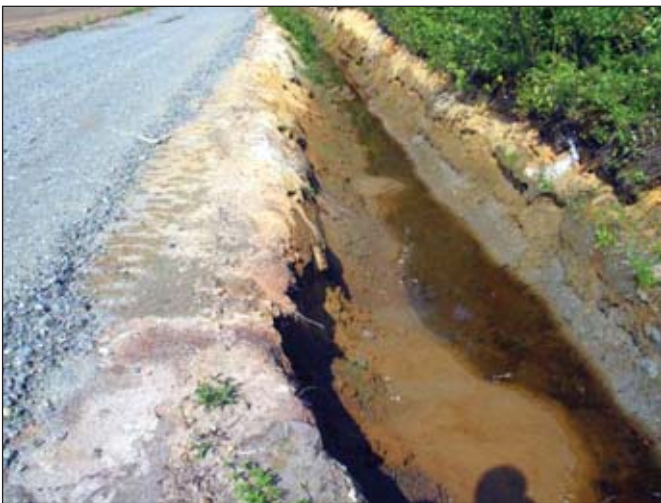
Photo 3: Piping caused by excavation of a stream in soil with an elevated water table Source: Victor Savoie, MAPAQ
