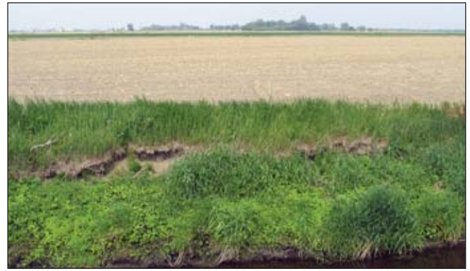
Photo 15: Bank failure. Source: Robert Beaulieu, MAPAQ
