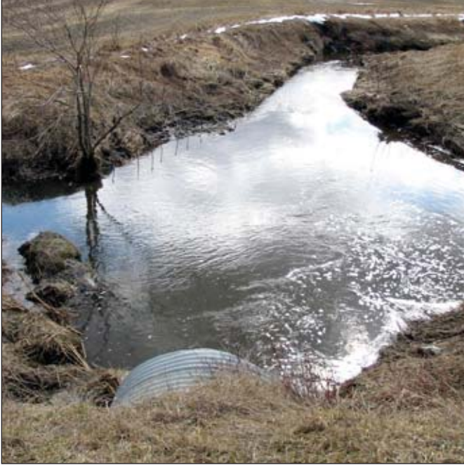
Photo 8: Widening of the streambed downstream of a culvert Source: Mikael Guillou, MAPAQ
