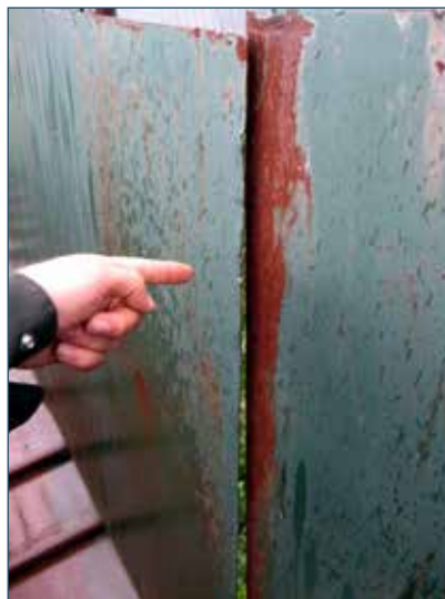
Figure 14. Example of a dangerous sheet metal joint
