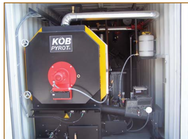
Biomass Boiler (Photo: Ian Pickering)
