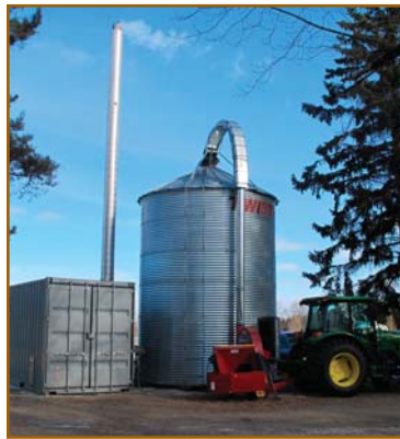
Biomass Heating System (Photo: Ian Pickering)
